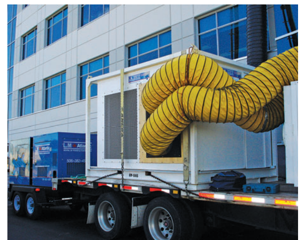
This temporary HVAC equipment is flushing the HVAC system at a Halifax LEED project.
